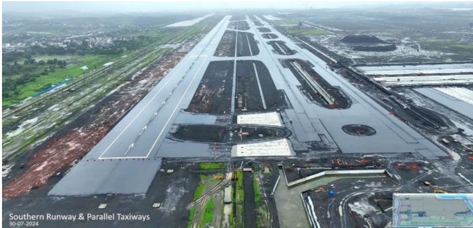
Southern Runway, Rapid Exit Taxiway, Drainage system completed, ILS26 Calibration test completed – July 2024
