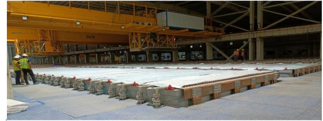
Refinery Cells commissioned
